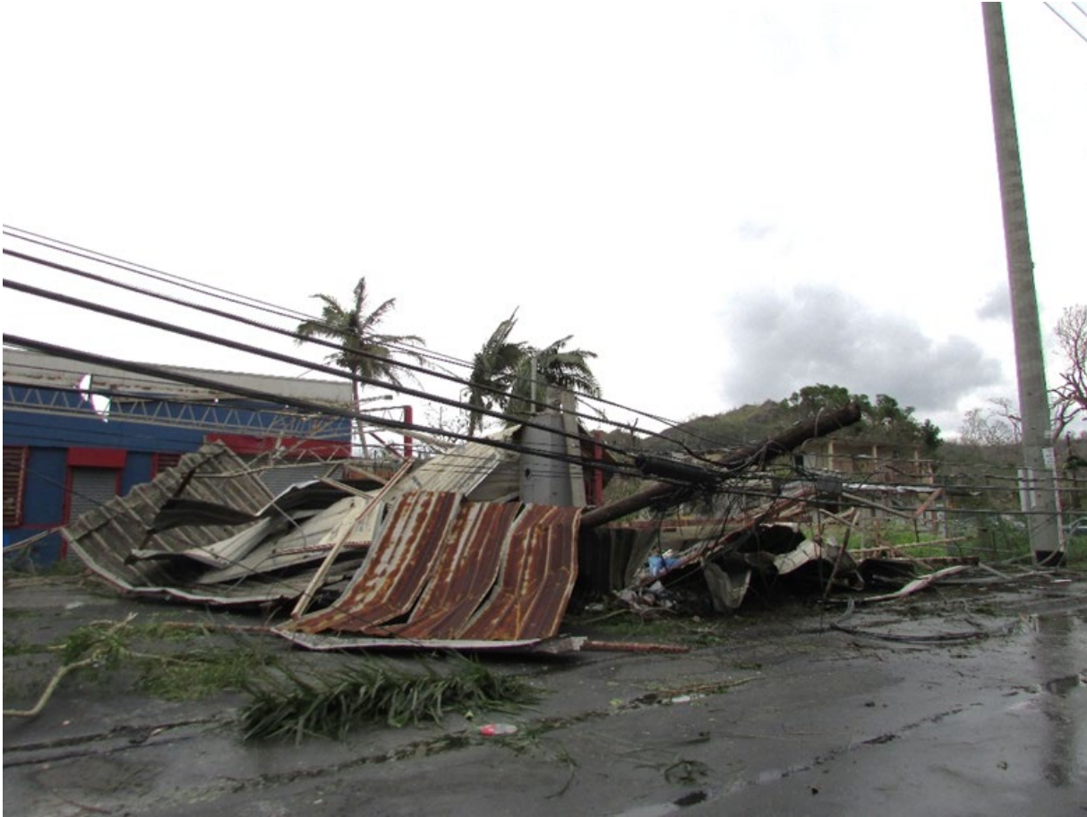
Figure 26 - Wooden electrical distribution pole damaged by Hurricane María at Trujillo Alto, Puerto Rico
