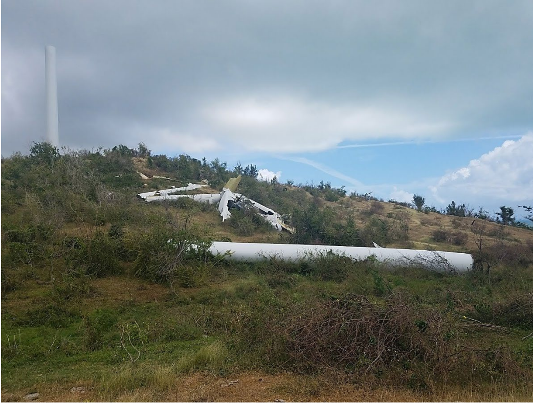
Figure 25 - Inoperable and damaged wind turbines at Punta Lima wind farm after Hurricane María in Naguabo, Puerto Rico
